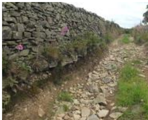
Photograph 8: Limer Rake, Staffordshire. Closed by a temporary TRO because of fears of walls collapsing. These have been undermined by green laning and subsequent water erosion. July 2015
