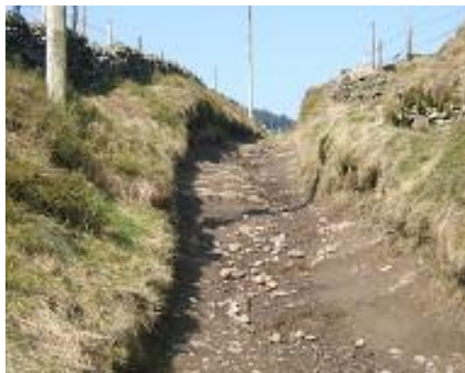
Photograph 1: Charity Lane, Cheshire: A UUCR where a narrow sunken lane without refuges shows the problem of meeting a green laning vehicle. March 2015
