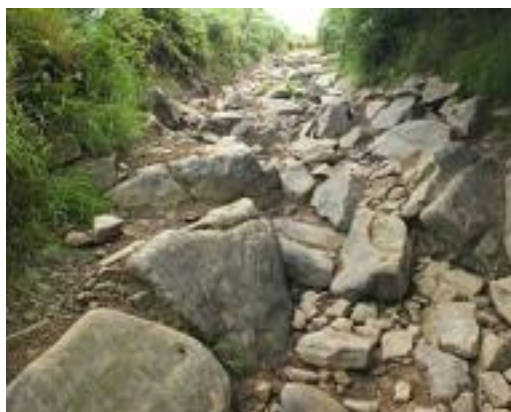
Photograph 9: Limer Rake, Staffordshire. Once a grassy path, the surface now makes the UUCR unusable for many non vehicle users. July 2015
