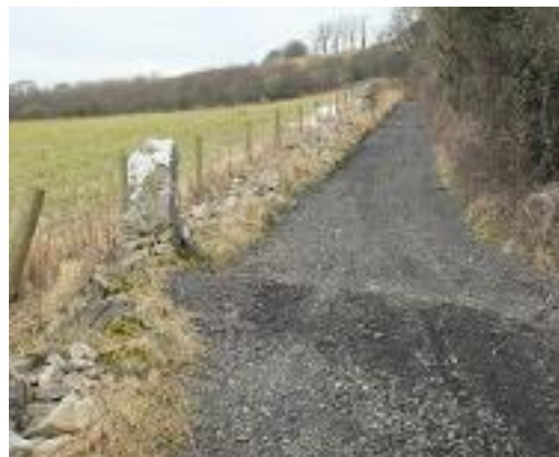
Photograph 6: Leys Lane, Derbyshire in February 2013 after DCC repairs. The dry stone wall was destroyed by green laners. Lane now protected by a TRO.
